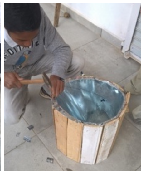
Securing the funnel onto the support. Each tab was trimmed and hammered. (photo credit RANO WASH)
