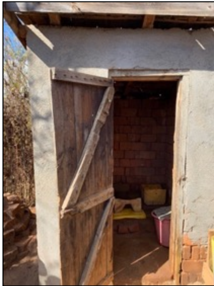
One of the latrines with a fly-proof cover. To the left of the latrine is the brick ventilation unit. (photo credit RANO WASH)
