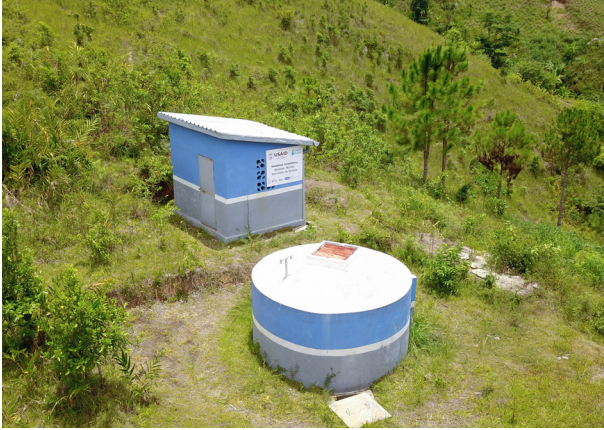
Infrastructure in Ambatofotsy (connection and tank)
