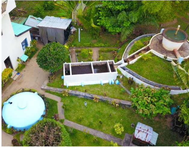
Aerial view of the Sandandrano offices with the surrounding drinking water infrastructure
